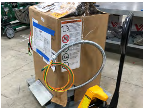
Transformer Prepped and Loaded on Setting System
